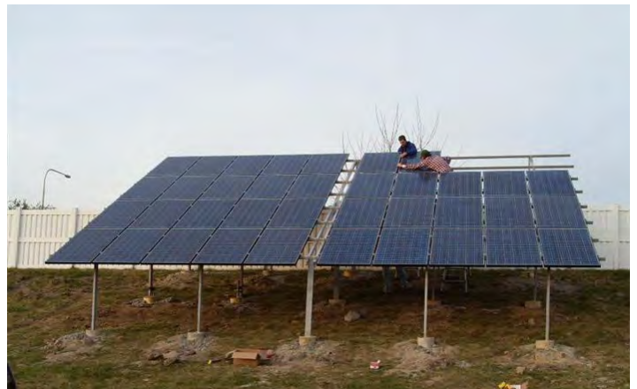
Solar PV panels in back yard.
