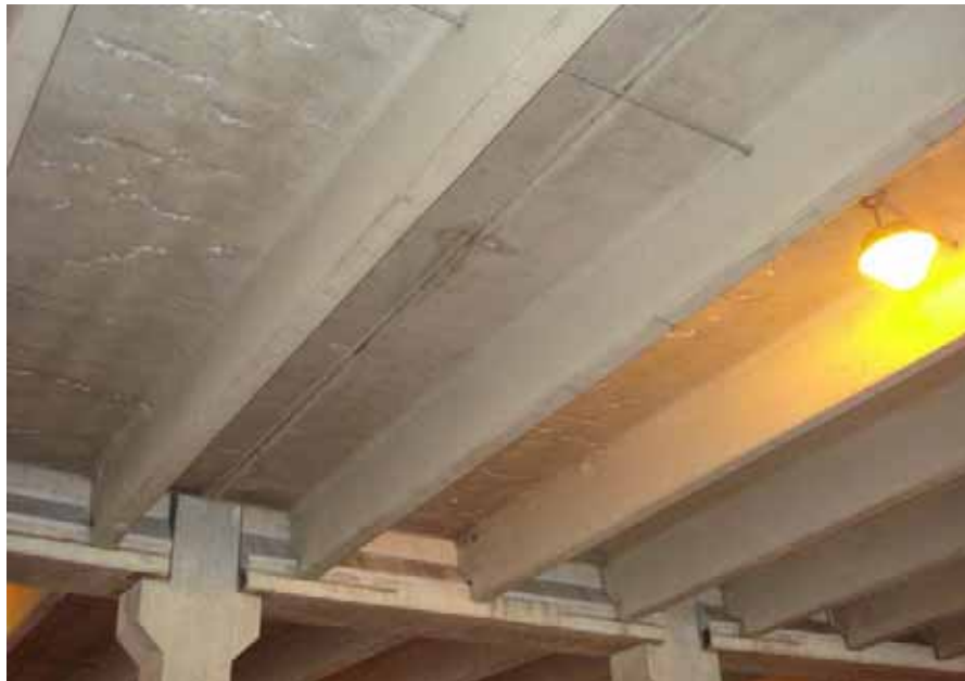
Joint issues and slab leaks in the Urbana parking structure.
