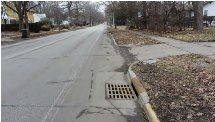
Figure 204 Transverse drainage grate, flush with the pavement, in the Washington Street bike lane east of Vine Street
