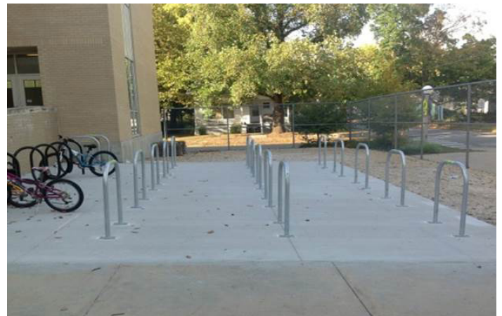
Figure 110 Inverted U bike racks on the east side of Leal Elementary School (Credit: CUPHD)
