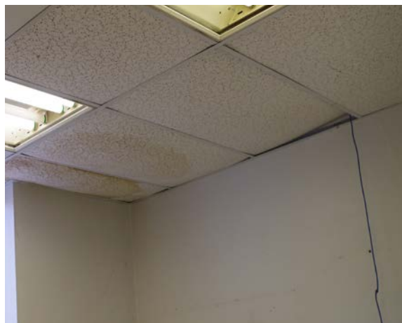
Right: Interior water damage at park building 901. (03/08/2016)
