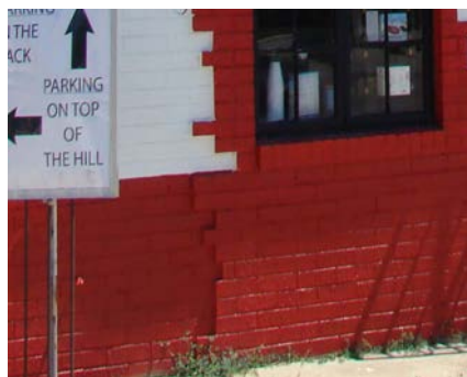
Above & Left: The exterior brick walls at 303 W. Main have severe step and sheer cracking.
