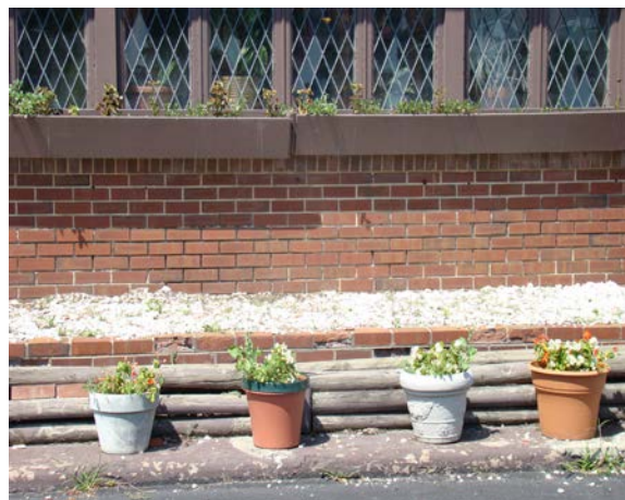
Right: 403 W. University is in need of tuck-pointing.
