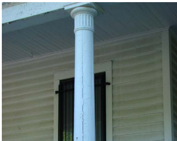
Left: The porch column at 206 S. Cedar is cracked.
