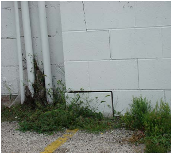
Left: Foundation settlement at 301 E. Main.
