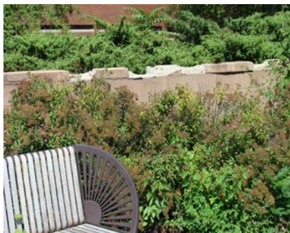
Above: This retaining wall located at 1776 E. Washington is cracked and crumbling.
