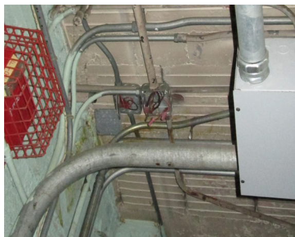
Right: Improperly terminated wires. (04/04/2016)
