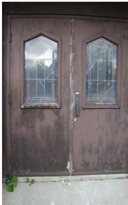
Right: A deteriorated door at 201 S. Race.
