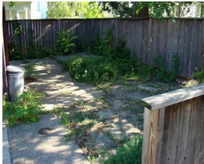
Above: The side lot at 202 W. Green has deteriorated pavement.
