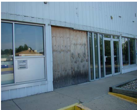
Left: Deteriorated siding and doors at 105 E. University.
