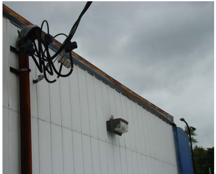
Above: The flashing and gutters at 501 S. Vine are rusted.
