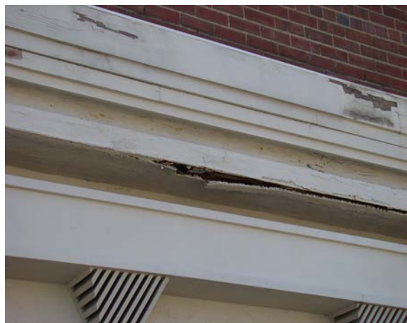
Left: Rotted soffit and fascia at 129 N Race.
