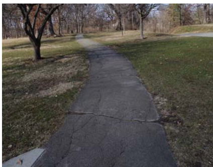
Left and Right: The pathway located in Crystal Lake Park is deteriorated. (03/08/2016)
