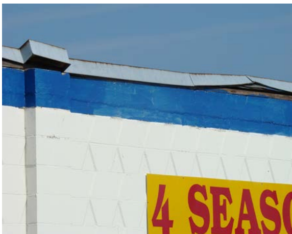
Left: Dislodged flashing at 401 N. Broadway.
