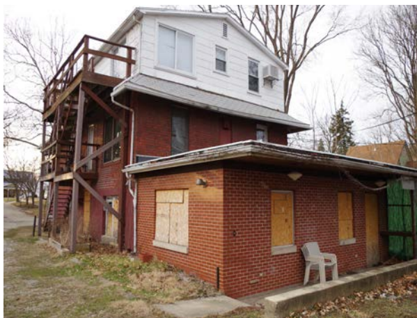
Right: 202 Wood is a deteriorated, boarded up multi-family apartment building with 1 occupied unit. This buildings has deteriorated siding, shingles and gutters. (03/07/2016)
