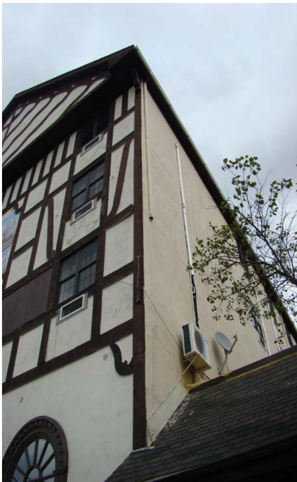
Left: A large portion of the downspout is missing at 201 S. Race.
