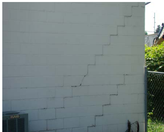
Right: Step cracking in the concrete block wall at 405 N. Broadway.
