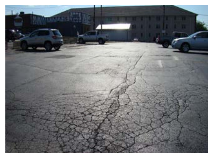
Above: The parking lot at 710 W. Florida Avenue has severe alligator cracking.
