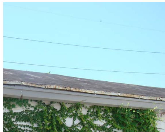
Right: The roof flashing on 302 N. Broadway is deteriorated.
