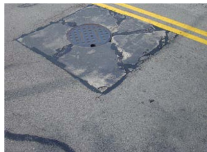
Below: The pavement around this manhole cover on Elm Street is deteriorated.
