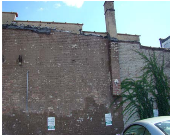
Right: The chimney and exterior brick wall at 201 N. Broadway are deteriorated.
