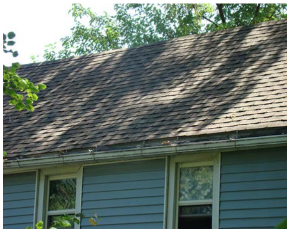
Left: The shingles on 404 N. Lake need to be replaced.
