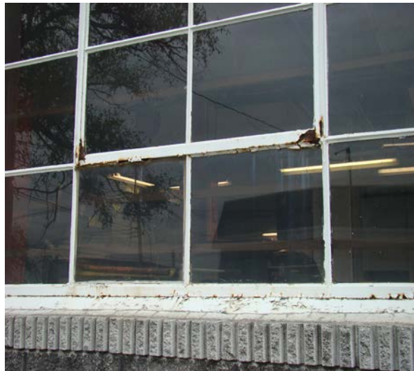
Right: The window muntins at 104 S. Vine are rusted.
