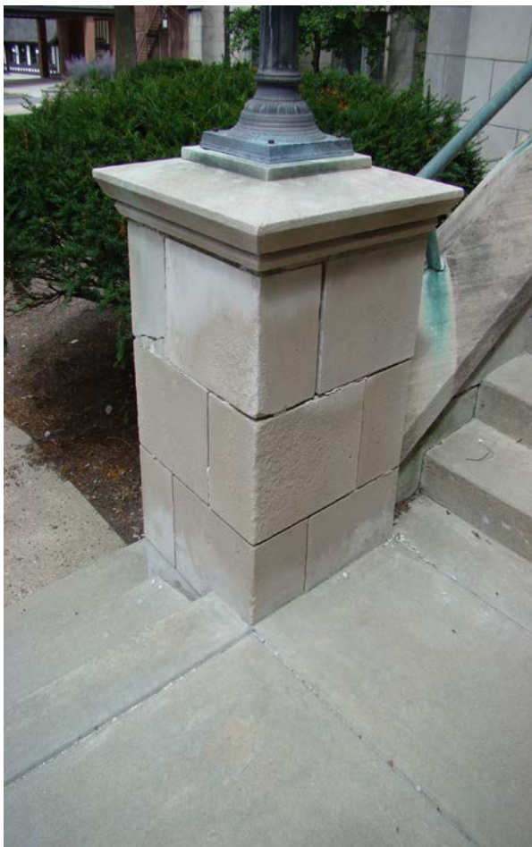
Left: The porch columns at 304 S. Race. are in need of tuck-pointing.
