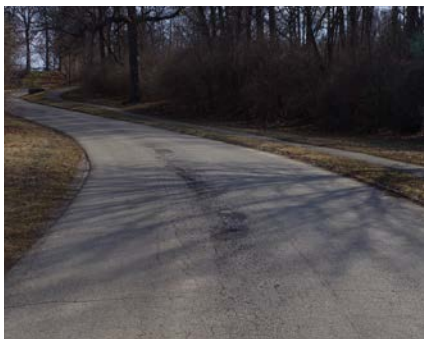
Left: The street pavement in Crystal Lake Park is deteriorated. (03/08/2016)
