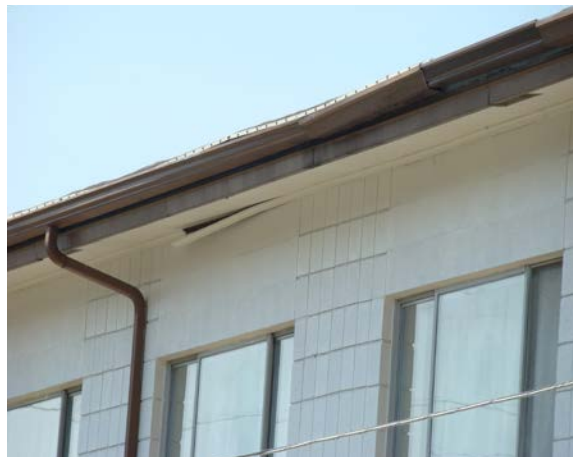
Right: 409 W. University has deteriorated gutters, soffit and fascia.
