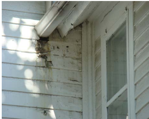
Right: The wood siding on 206 S. Cedar has rotted due to water leaking from the gutter.
