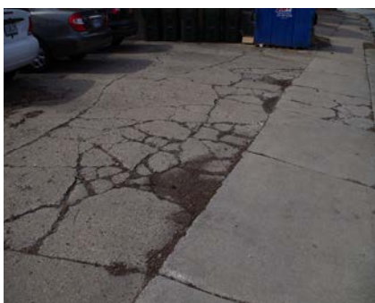
Left: The concrete parking lot at 101 W. Park is cracked and severely deteriorated. (03/08/2016)
