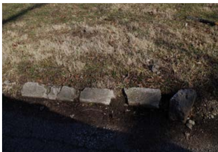
Left and Right: The curbs and gutters in Crystal Lake Park are deteriorated. (03/08/2016)
