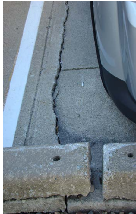
Above: A large shear crack, due to excess settling at 207 W Elm Street.
