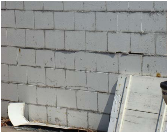
Left: Deteriorated mortar joints in the concrete block walls at 401 N. Broadway.
