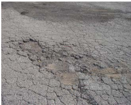
Left and Right: A deteriorated parking lot and curb stop located at 1501 N. 12th Street.
