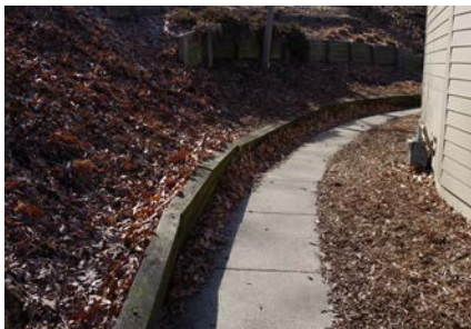
Left and Right: A leaning retaining wall located at Crystal Lake Park. (03/08/2016)
