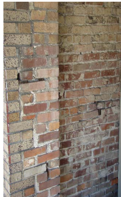
Below: Another example of the needed tuck-pointing at 110 W. Main.
