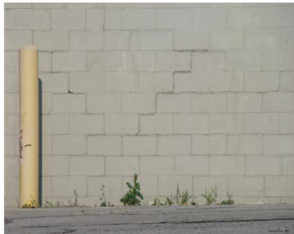
Right: Step cracking in the concrete block wall at 220 N. Broadway.
