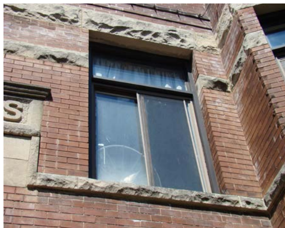
Left & Right: Deteriorated brick walls and windows at 218 W. Main.
