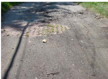
Below: This alley between Vine Street and Urbana Avenue is severely deteriorated.
