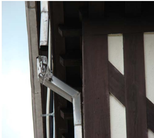
Above: A downspout at 201 S. Race has been dislodged.
