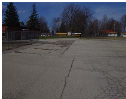
Low Right: The concrete parking lot at 410 W. University is cracked. (03/08/2016)
