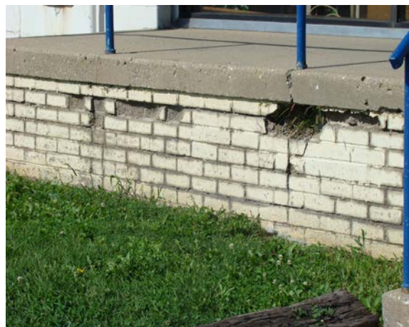
Right: A deteriorated brick front entry at 401 N. Broadway.
