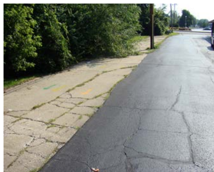
Above: The pavement along Courtesy Road is deteriorated.
