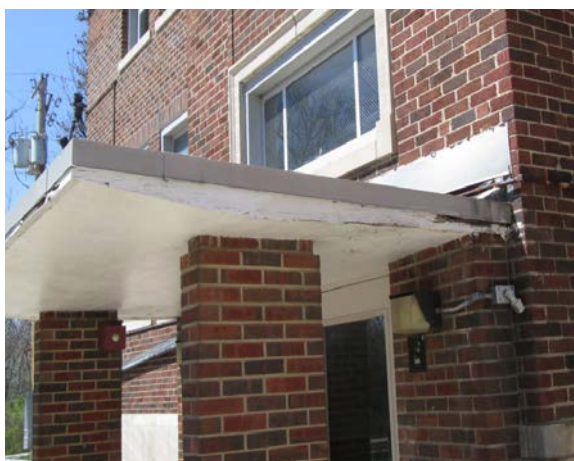
Left: The exterior awning is deteriorated with rotted framing. (04/15/2016)
