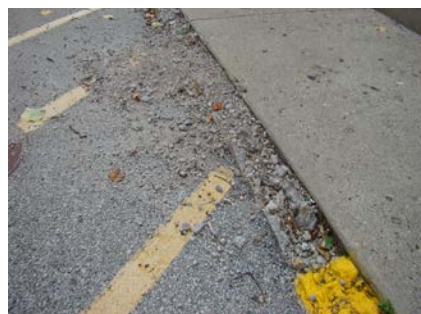
Below and Right: Crumbling curbs and pavement located at 202 S. Broadway.
